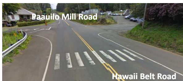
Existing faded crosswalk at Paauilo Mill Road, looking south.
